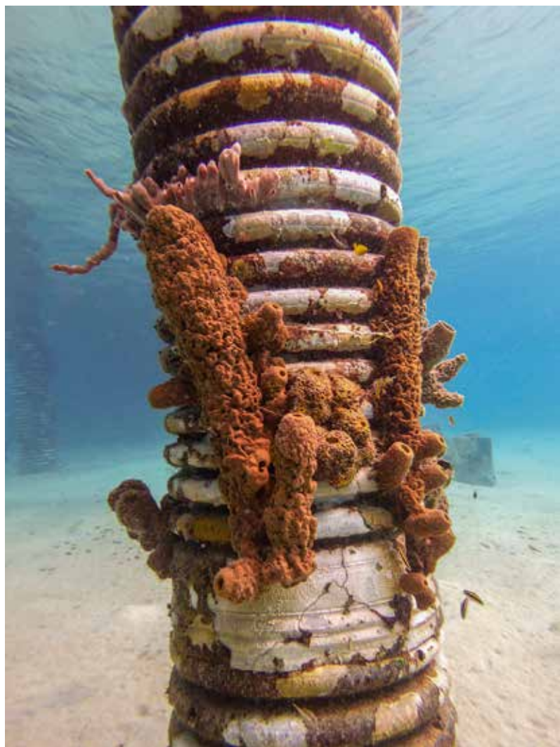
If you were looking at this piling in person, you'd be able to see more clearly how the sponges are sort of absorbing the fishing line which was used to attach them. The large tube sponge on the left has already grown several new tubes.
