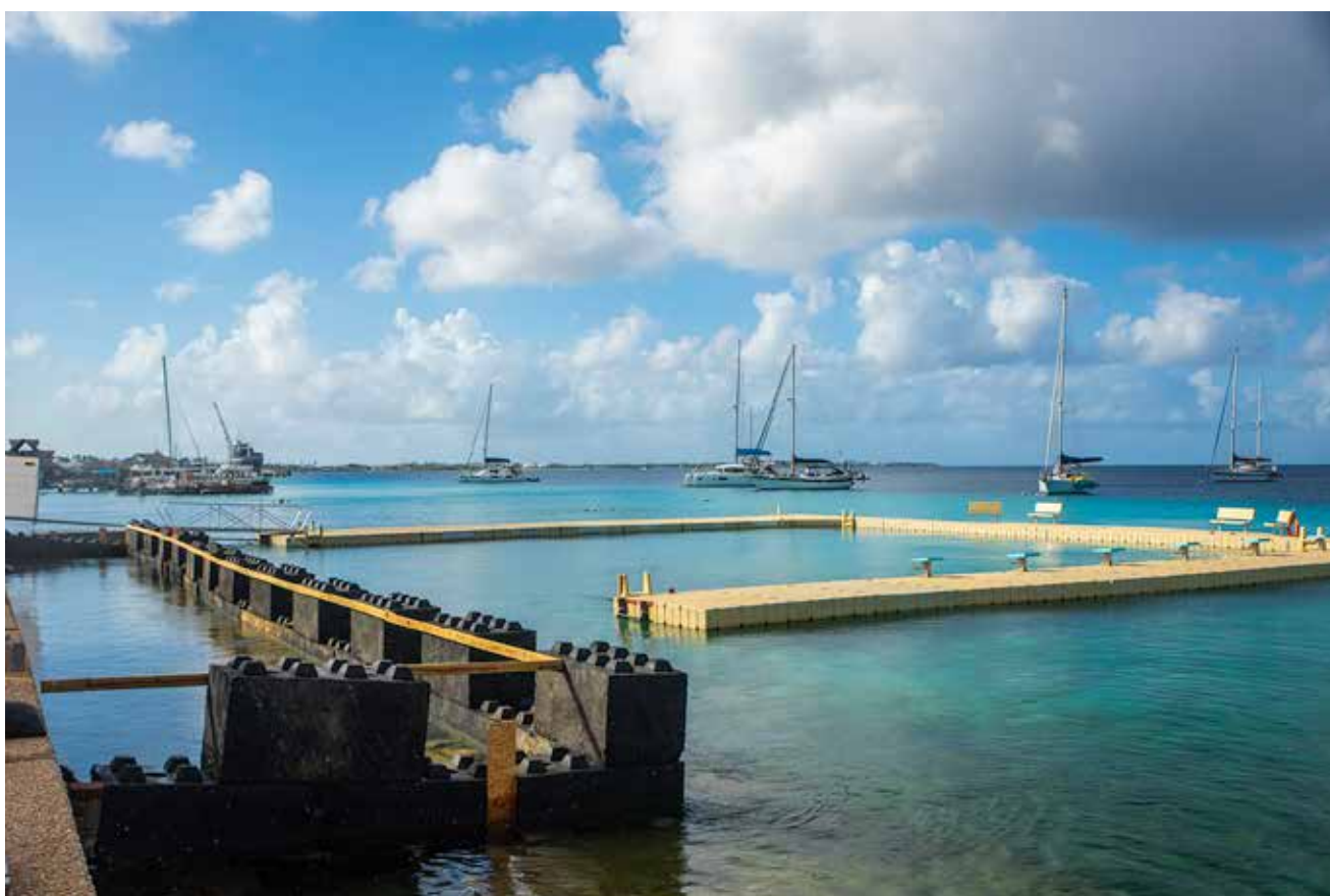
STINAPA is building an access ramp for people with disabilities at the floating swimming pool at Parke Tului. The work is expected to be completed before Christmas. DMR
