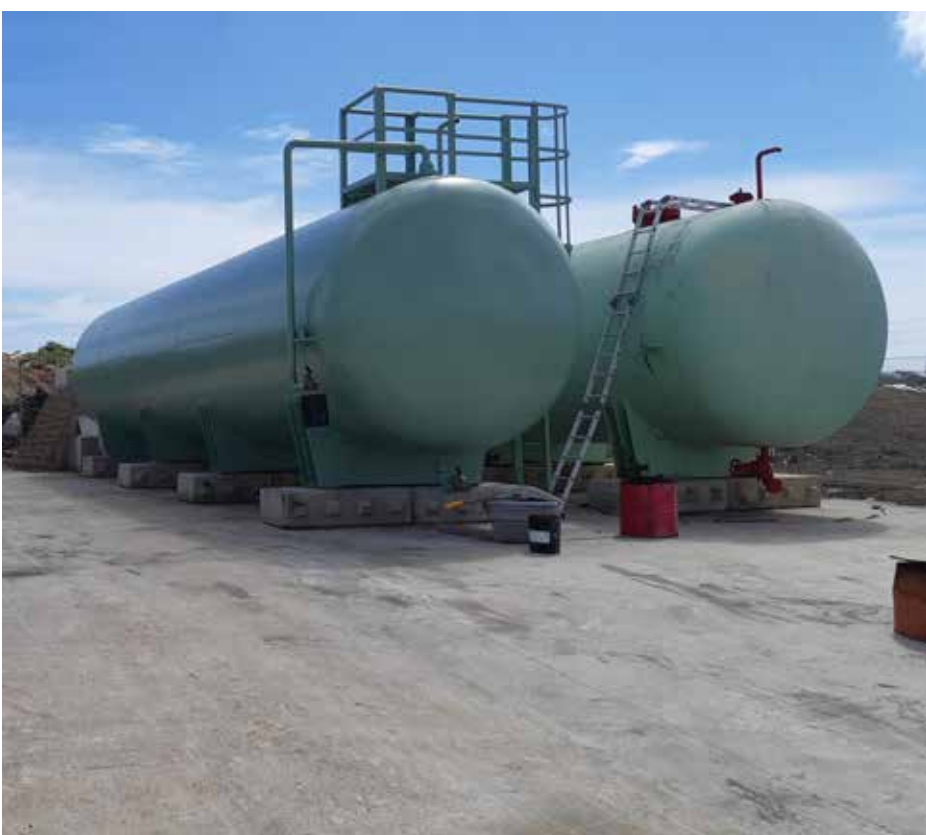
Selibon's new oil tanks
