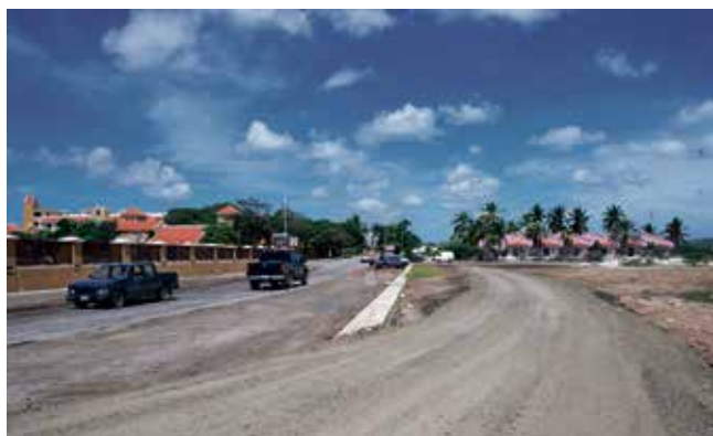
The Spatial Planning and Development Department of the public body of Bonaire constructed a temporary dirt road on Bulevar Gobernador Nicolaas Debrot. The temporary road was built to combat the seawater that often floods the road in the bend at Harbor Village Marina Bonaire.
