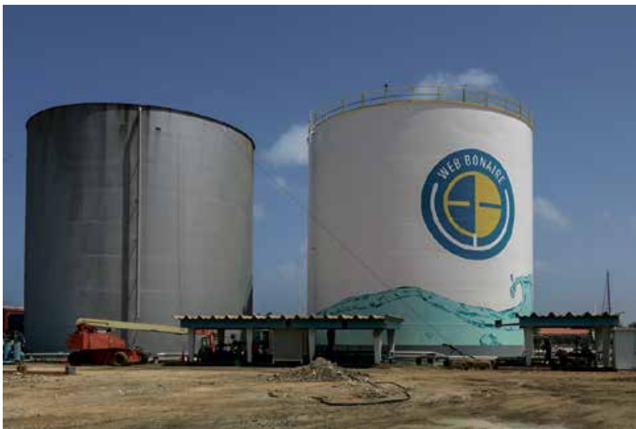
Water and Energy Company Bonaire (WEB) is on schedule with maintenance work of Hato's water storage and distribution tanks. One of the water tanks has been completed and is fully operational. It has a special paint job that can be seen from far away. The design was painted by hand, in a period of four weeks by the artist Loes Praagman. Maintenance work started in July 2019. Periodic maintenance is necessary in order to comply with the Electricity and Drinking Water Act BES and to guarantee security of supply.
