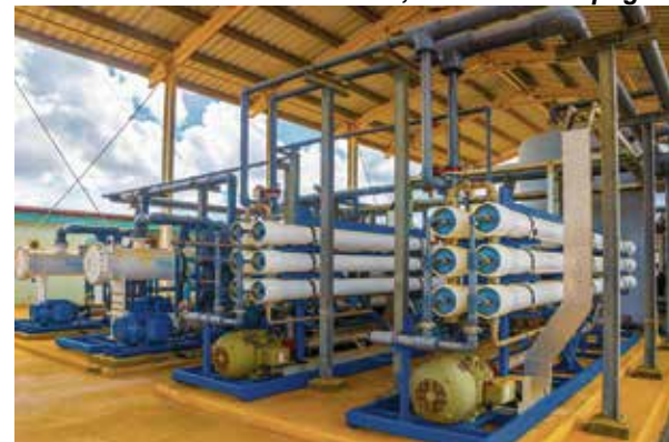
WEB and GE current reverse osmosis system provides 1600m3 and 4800m3 respectively per day.
