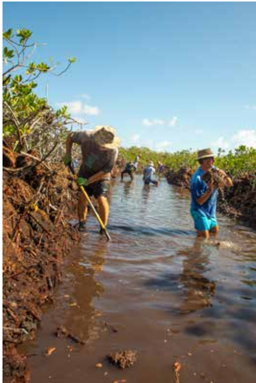
Mangrove Maniacs cut and dig a pathway to the sea with shovels and saws to provide fresh sea water to the mangroves.
