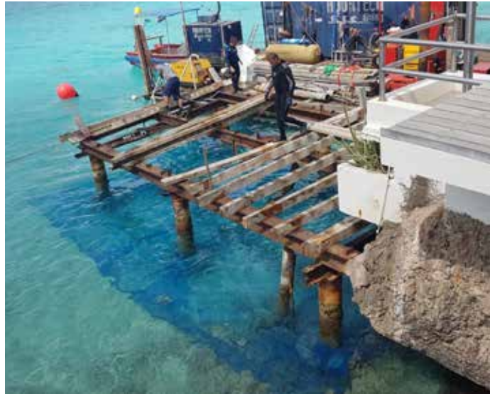
A net is placed below the pier construction to catch any falling objects that could contaminate the water and prove hazardous to marine life.
