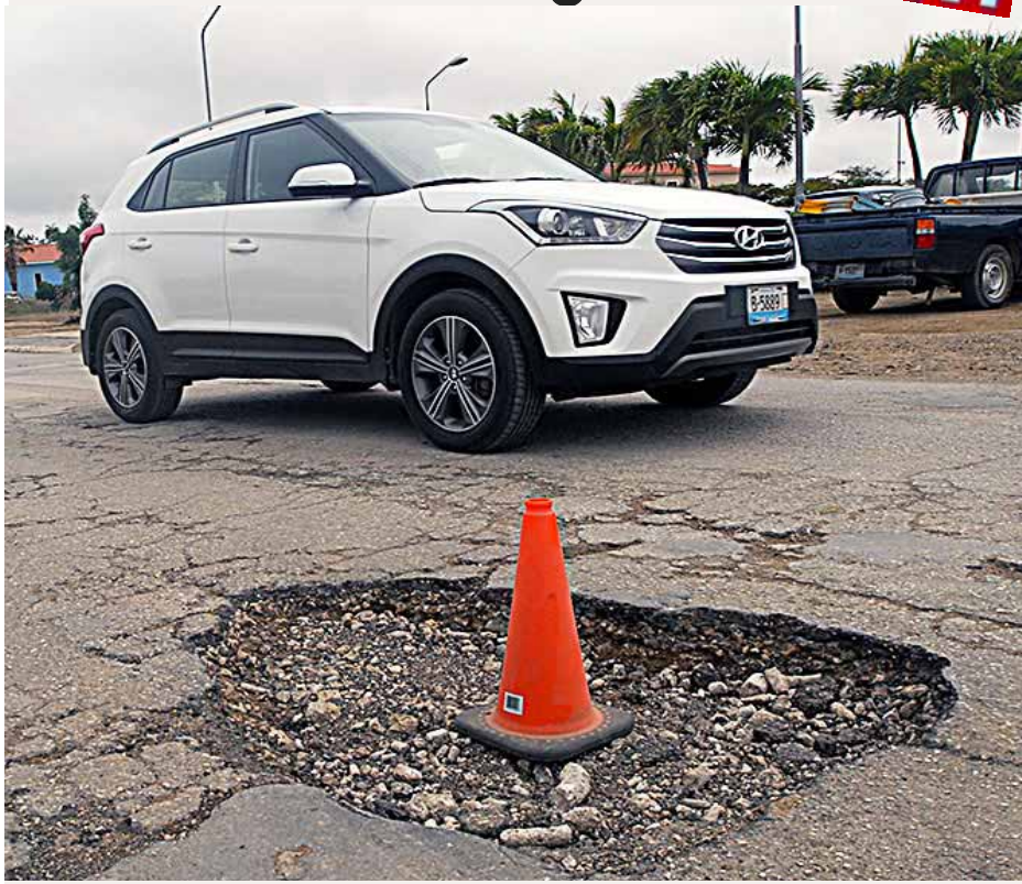
This pothole was temporarily repaired with “diabas” over a bed of crushed stone. It washed out in the next rain but was promptly repaired the same way.
