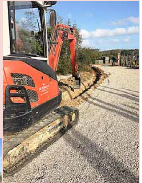
A trench is dug to support the curbs that border the road. Watch out for buried pipes and wires.
