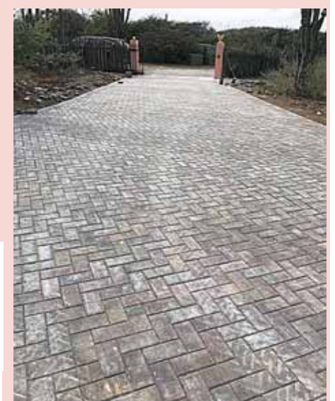
Finally complete with multi-colored paving bricks. All that remains is rain to wash the sand away
