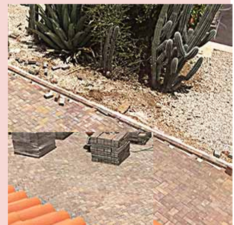
The curb is a critical element. There are straight or curved sections
