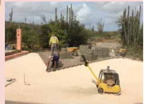
After the surface is prepared, the spread sand is compacted. The bricks are laid atop the sand
