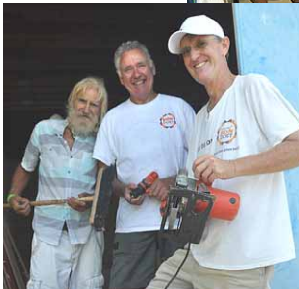
Volunteers build shelves at the Animal Shelter's flea market, Paskus di Pruga.
