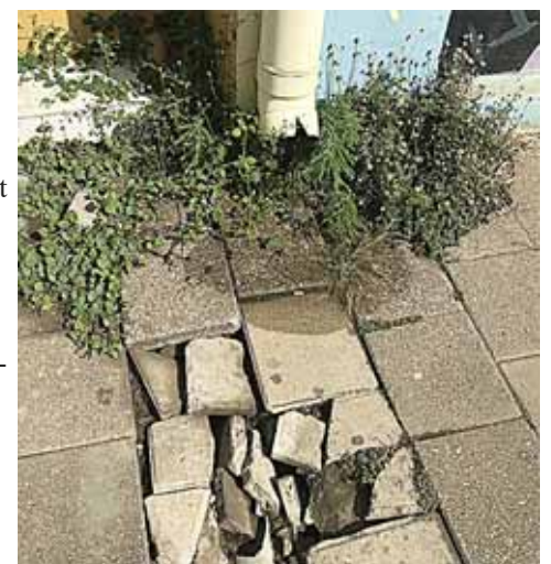
Some sidewalks have been so long without repair that verdant gardens are growing.
