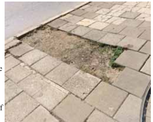
However, the sidewalks are often so broken that rolling a wheelchair is a big problem
