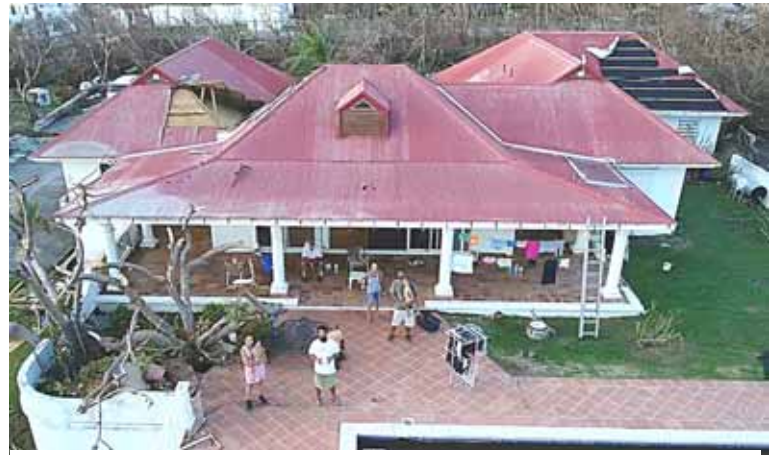
We rode out the storm in this house. Notice the damage. We are standing out front -safe.
