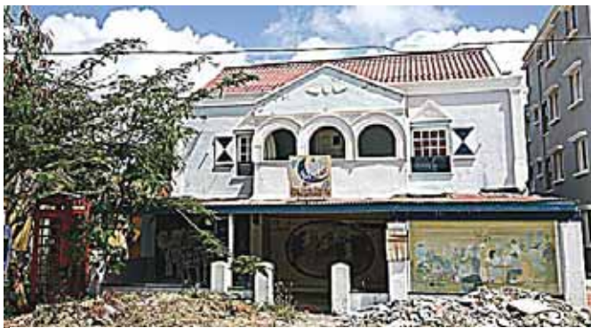
The demolition of The Blue Moon Restaurant on the waterfront. It formerly was Chez Truus. Now a condo/apartment building occupies the site.
