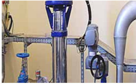
Vacuum Sewer Lines
