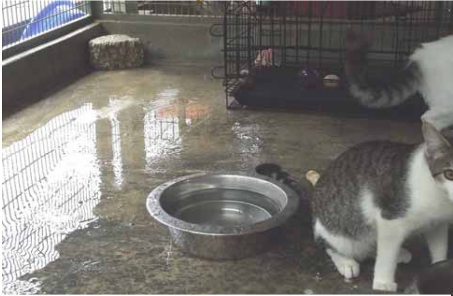
Despite routine maintenance, repairs and modifications, the cat compound can barely survive another rainy season. When the rain finally stops, the compound remains wet and damp for hours. But it is a space that the shelter cannot afford to lose until something else is available.
