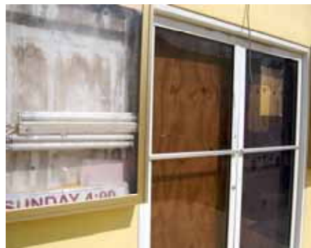
Boarded up doors are all that's left
