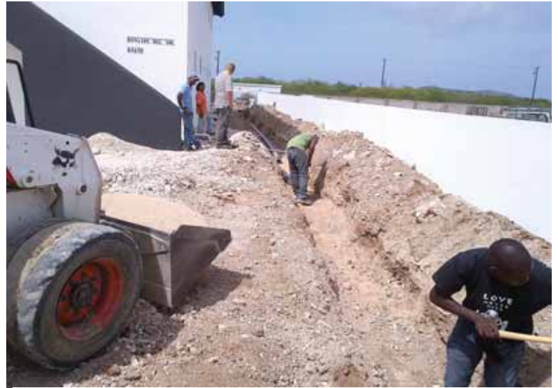
A trench must be dug from the house drain pipe to the sewer line
