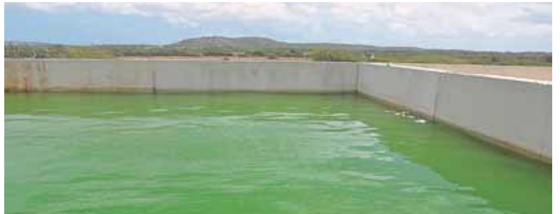
A water test in one of the treatment tanks
