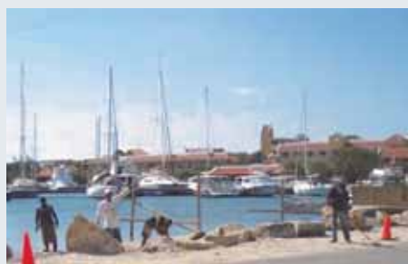
Workers closing the HV small boat ramp. High priced slips have replaced it.
