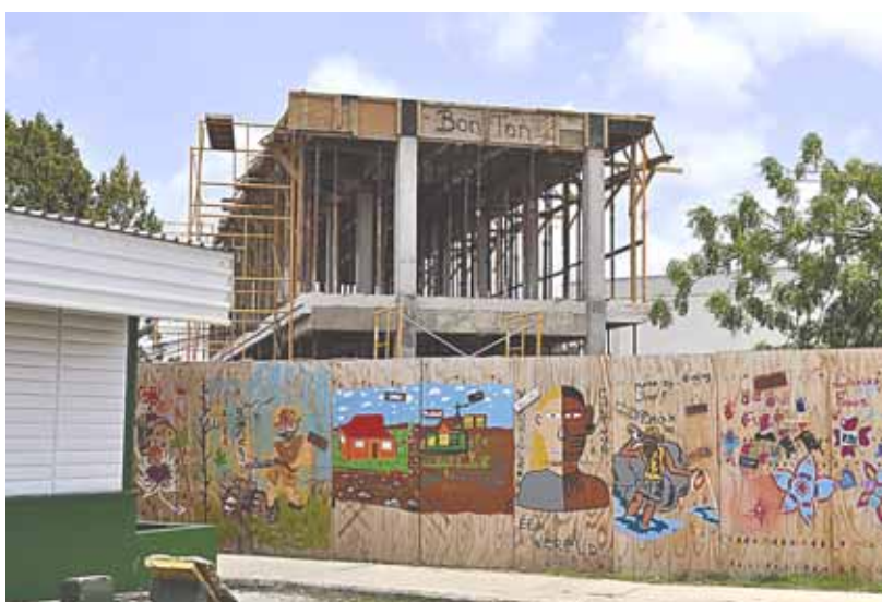
The unfinished school building – paintings on fence were done last year by the students for Cultural Week
