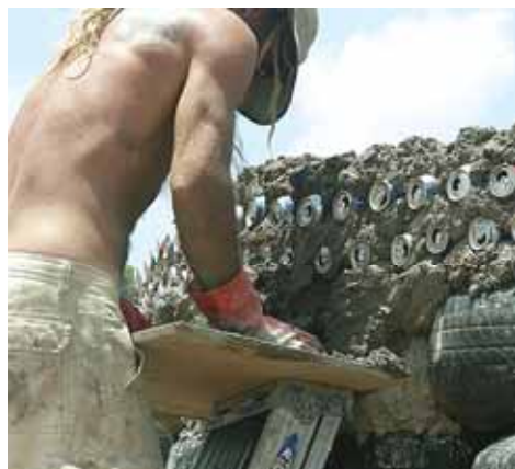
A worker setting the mortar into the tire/beer can matrix by hand
