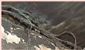
Electrical wiring was thought to be the fire's cause
