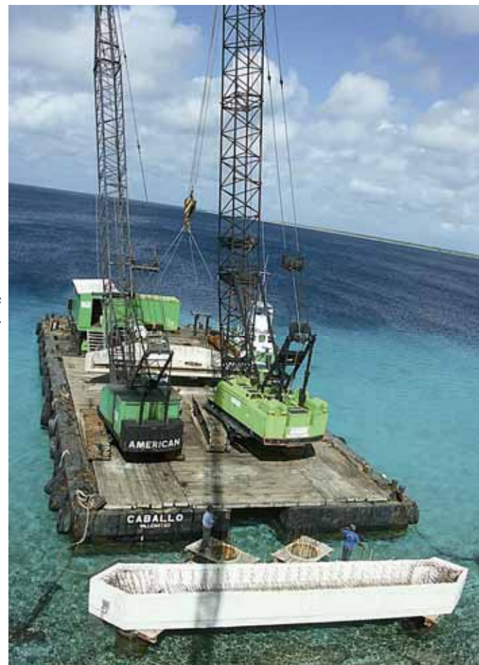
Three huge construction cranes are being used to install the mooring dolphins inshore for the South Pier. The base for the dolphins is in the foreground
