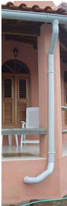
Gutters can catch rain from the roof to store in a cistern or barrels
