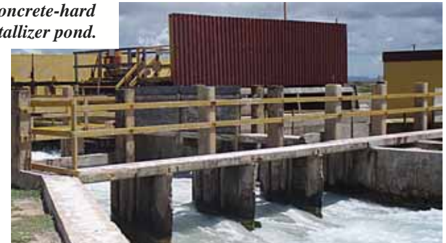
Electric pumps maintain proper flows and levels. Works water flow is from east to west
