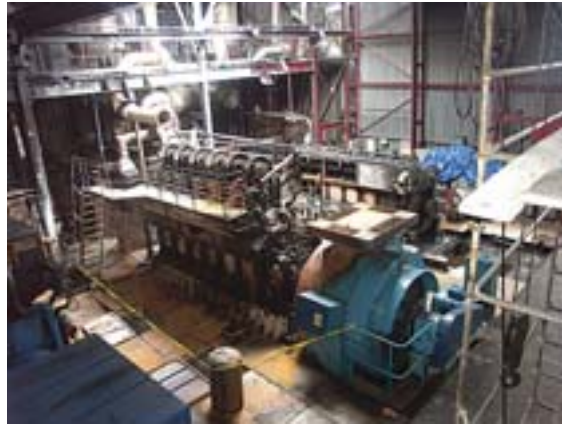
In February 2005, the WEB powerhouse at Hato was severely damaged by a fire that cut WEB's electrical power production by 40%-50%
