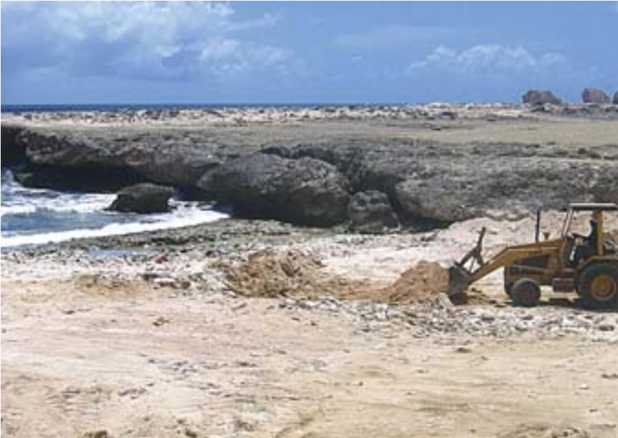
A loader removes sand from the beach at Onima in August 2005. STCB photo
