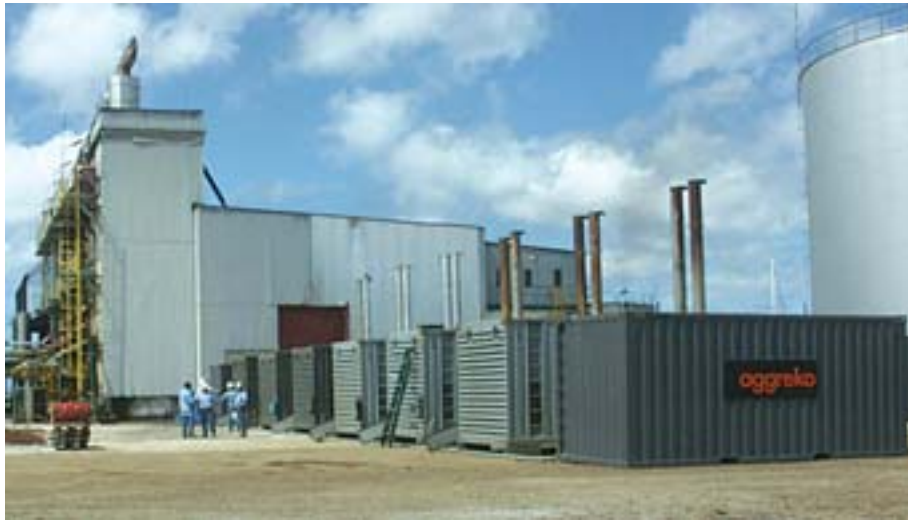
Aggreko generators being set up on the WEB property
