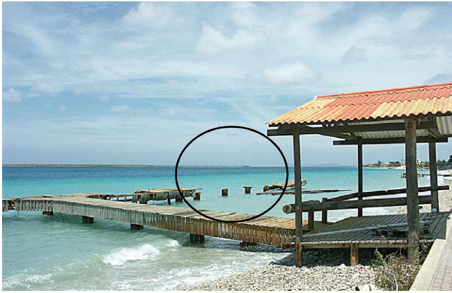
The Fisherman's Pier broke up when the supports broke off the rusted bases. The bases were relatively new.
